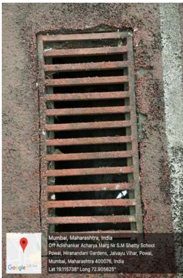
Channels for collecting rainwater and excess gardening water
