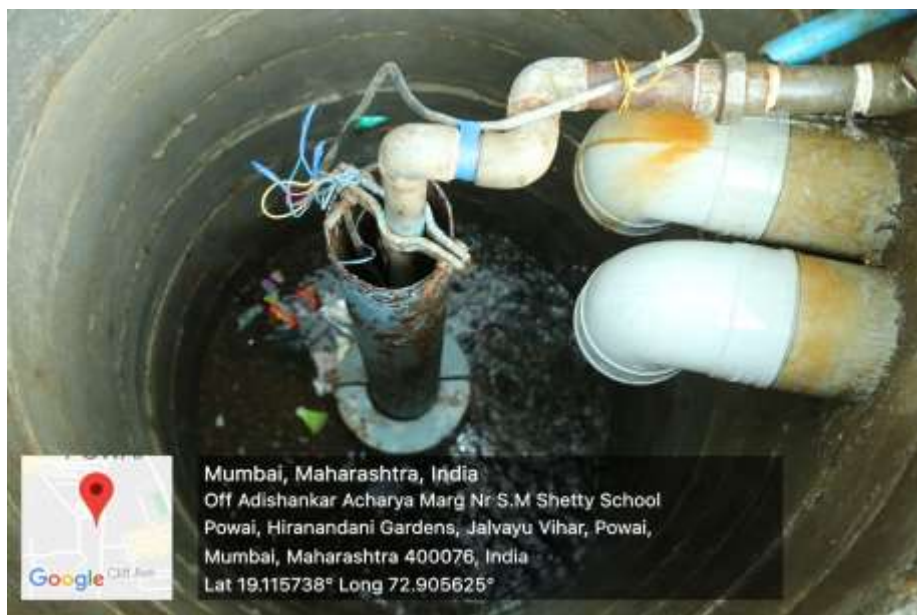
Waste water collection for cleaning by filtration system
