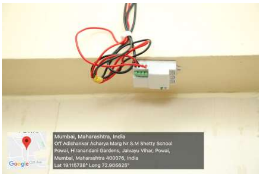
Sensors at the entrance of Staff Washroom
