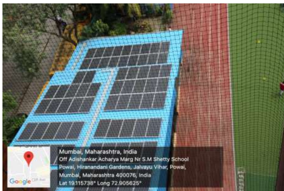
Aerial view of Solar Panel
